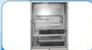
Battery back-up: Emergency power supply
